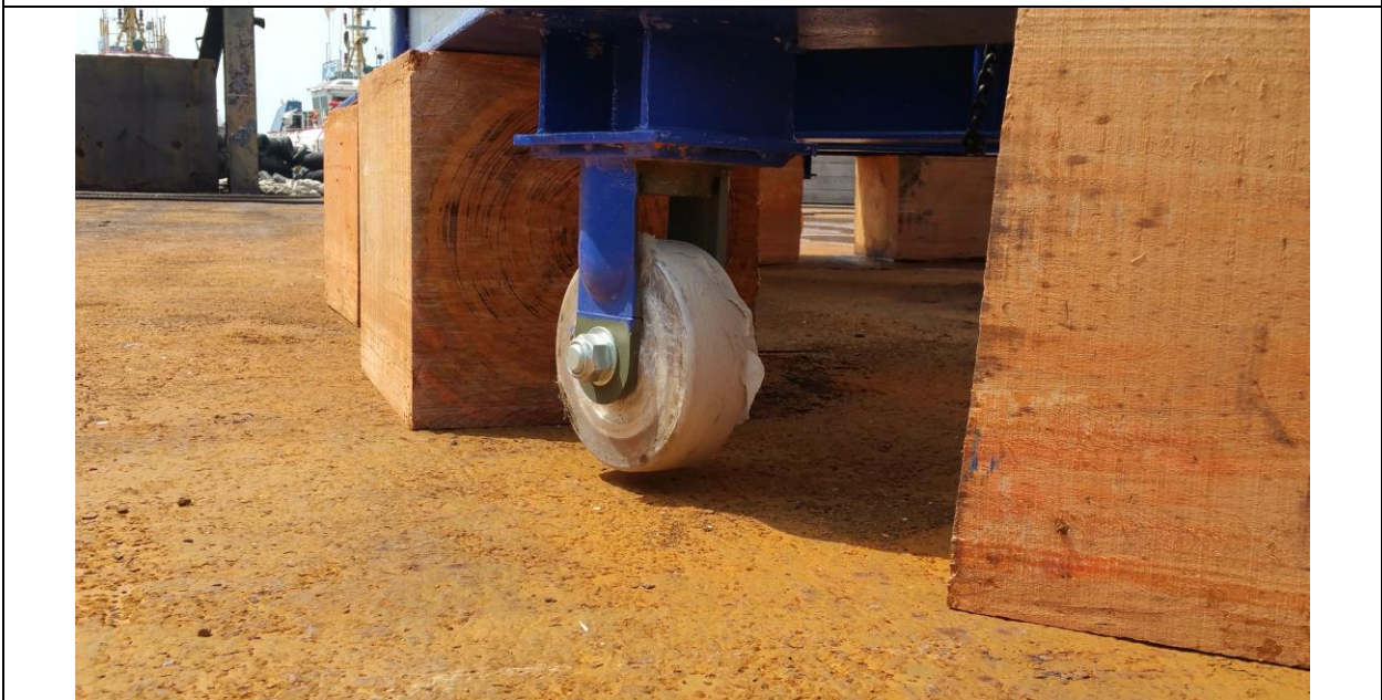
Pic 3: View of wooden blocks jacking up the production jumper, with rollers free from barge deck/ground
