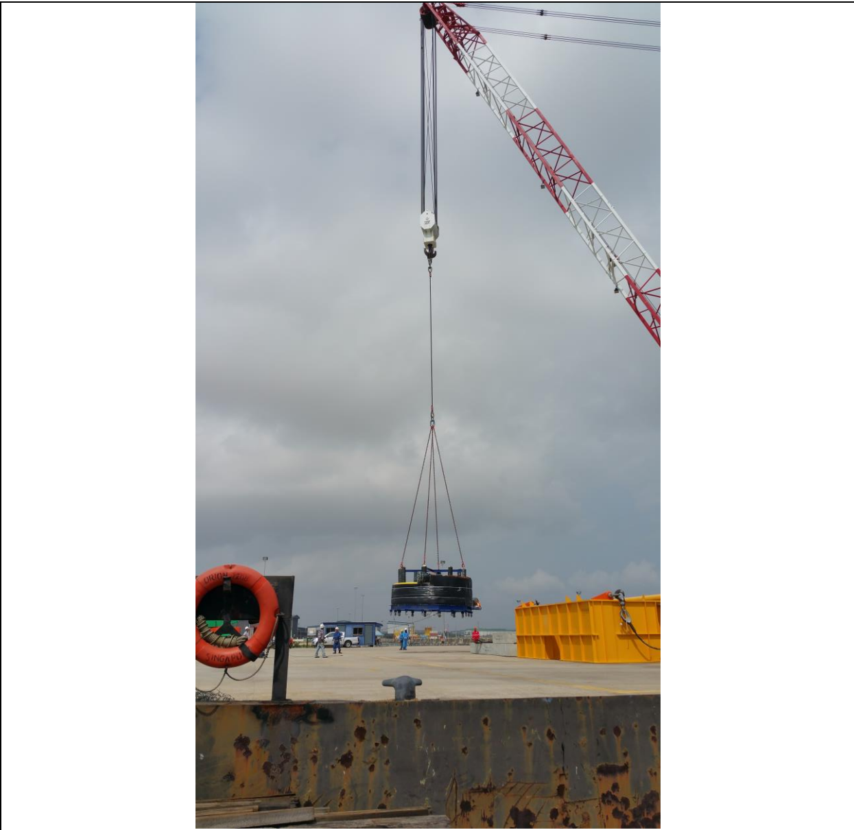
Pic 1: 1x unit production jumper at dim: 5.50 meter dia x 3.13 meter, weight: 21 ton. Loading onto barge using crawler crane in Tanjung Langsat, Johor Malaysia
