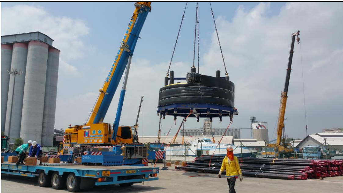
Pic 5: Mobile crane off-loading cargo from trailer onto ground for short term storage, pending for connecting vessel to Australia
