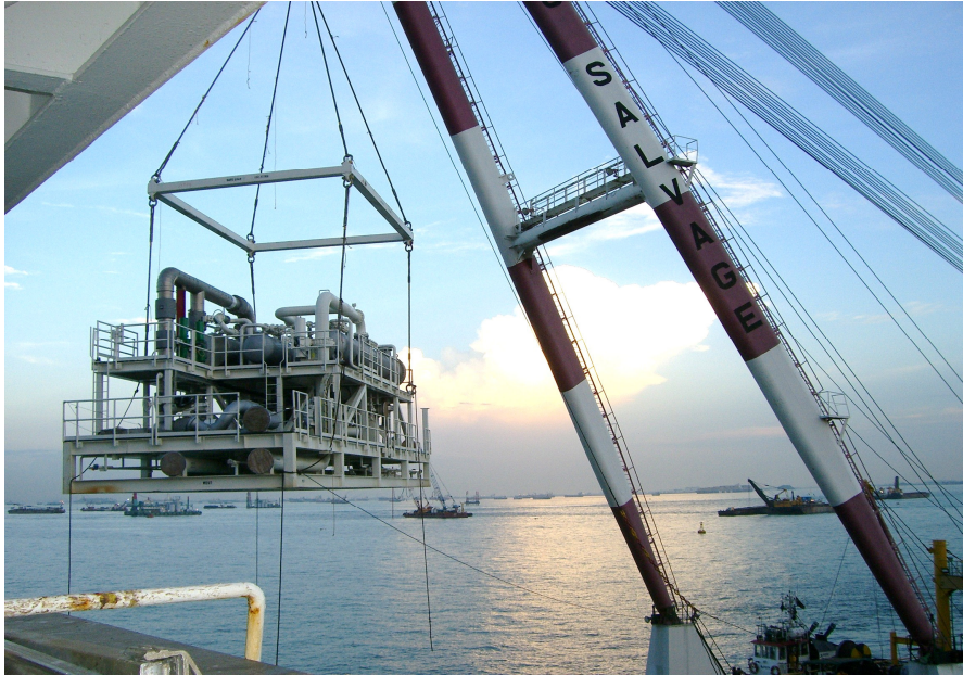
Transportation of Module Dehydrators loaded onto Barge Winstar II (180ft x 50ft x 10ft)
