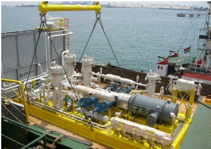
The Gas Compressors are discharged to Rickmers Jakarta
